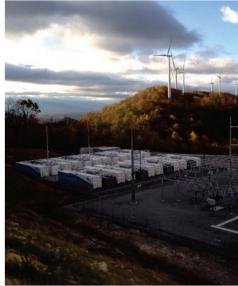
32MW storage system at AES Laurel Mountain wind generation facility is the largest lithium ion battery project of its kind in commercial operation
