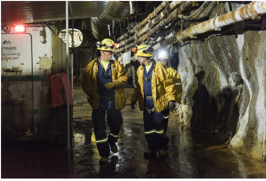
Pumps remove 600 gallons of water a minute from Resolution's No. 10 mine shaft. PHOTO: MARK PETERMAN FOR THE WALL STREET JOURNAL
